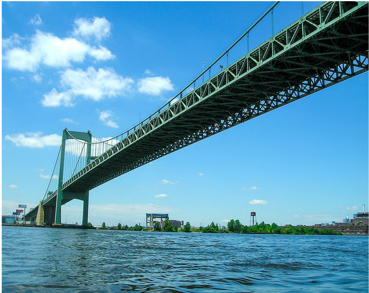
The Walt Whitman Bridge over the Delaware River, Philadelphia, PA to Gloucester City, NJ Photo from a Kayak, looking towards New Jersey, June 11, 2010, Courtesy Jag9889, Wikimedia Creative Commons Attribution-Share Alike 4.0 International License
